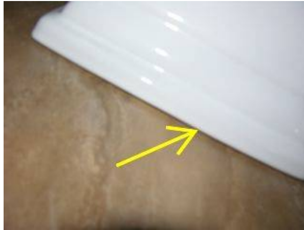
Photo 40-2 Caulking missing at the base of the toilet
