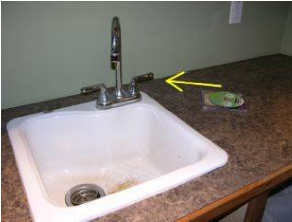
Photo 34-1 Back splash missing in the upstairs kitchen.
