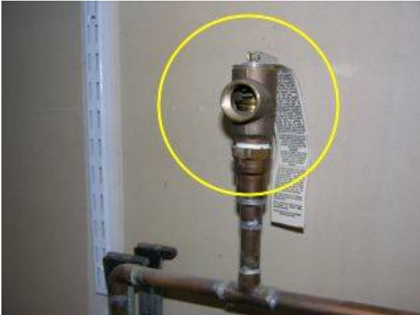
Photo 21-1 TPR valve missing piping.
