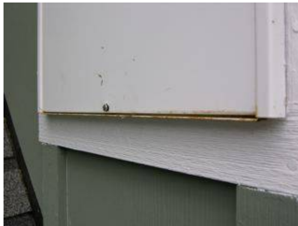
Photo 26-2 Bottom of the tankless water heater cover corroded. Unable to open.
