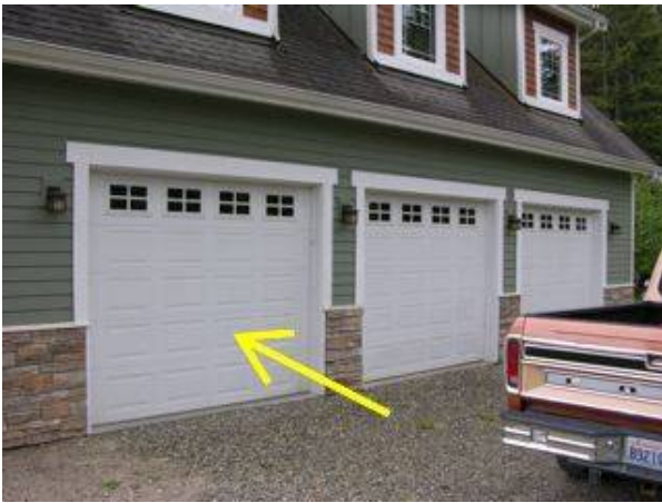
Photo 12-1 Left door (viewed from the outside) failed the midway auto reverse test.
