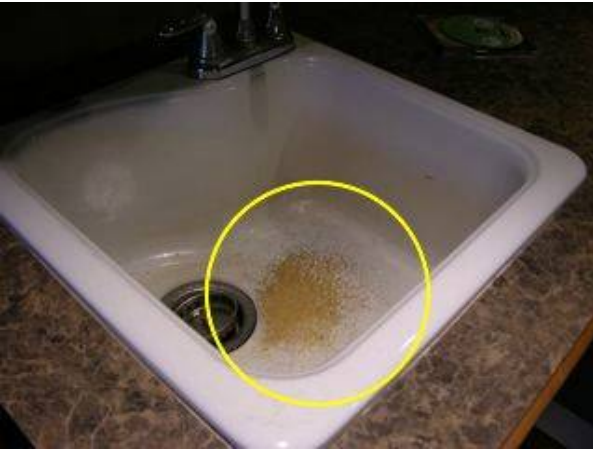
Photo 36-1 Damaged kitchen sink (kitchen above the garage)
