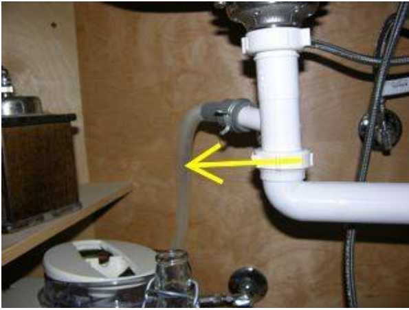
Photo 32-1 Dishwasher drain missing air gap or high loop
