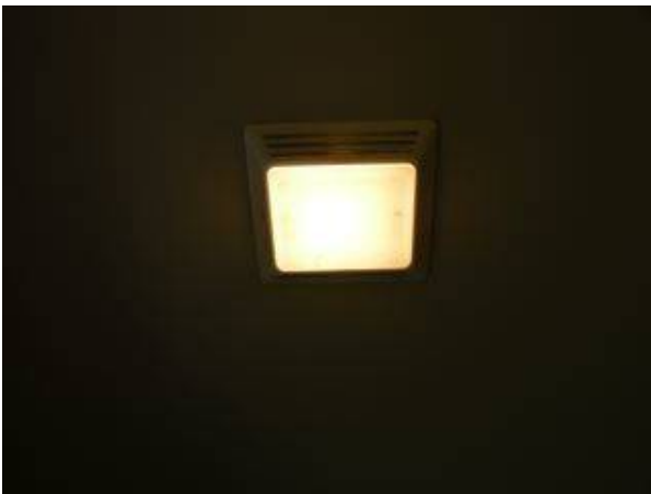
Photo 38-1 Fan in the bathroom located over the garage is noisy.
