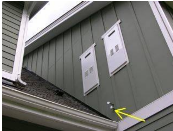
Photo 22-2 Hot water can discharge to persons below.
