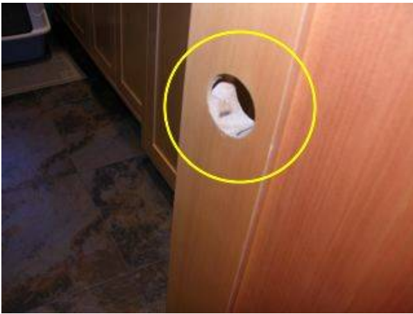
Photo 46-1 Laundry room door missing hardware
