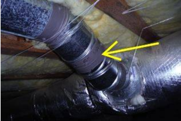
Photo 27-1 Heating ducts in the crawl space missing insulation
