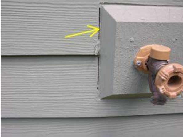
Photo 3-1 Needs additional caulking
