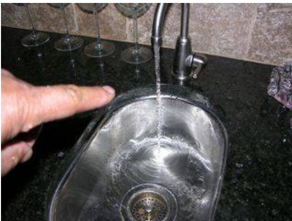
Photo 39-1 Faucet is loose.
