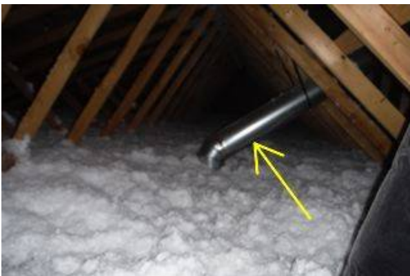
Photo 9-1 Exhaust ducts in the attic not insulated.
