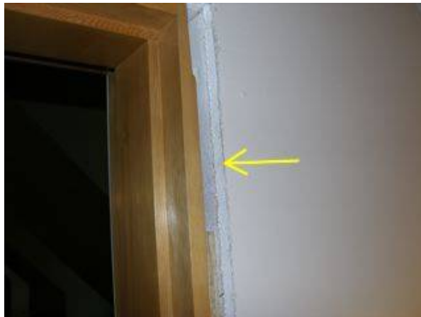
Photo 48-2 Missing door trim.
