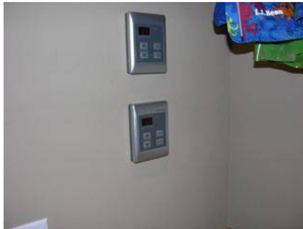
Photo 25-2 Remote controls for the Rinnai water heaters located in the laundry room.
