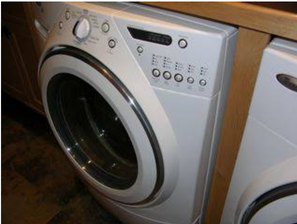
Photo 41-1 Under counter washer and dryer.
