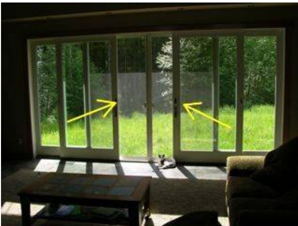
Photo 47-1 Sliding glass door difficult to open and close.
