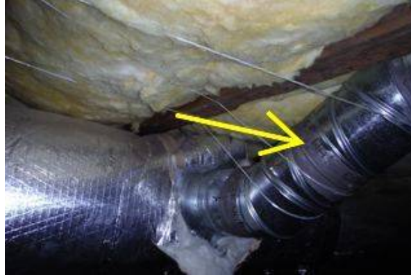
Photo 27-2 Heating ducts in the crawl space missing insulation.
