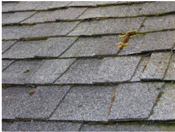
Photo 8-2 Moss growing on the roof. May require treatment.
