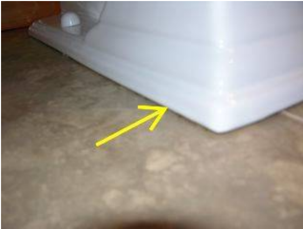
Photo 40-1 Caulking missing at the base of the toilet.
