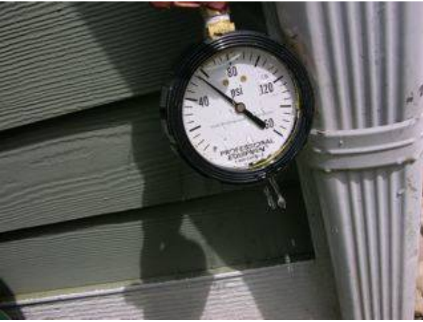
Photo 18-1 Hose bib leaked while under test.
