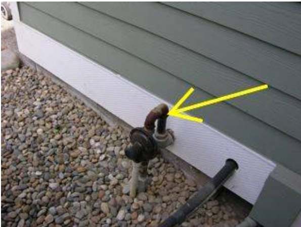
Photo 17-1 Corroded steel gas piping on the exterior of the residence.
