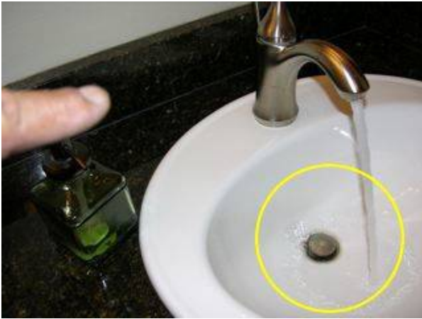
Photo 42-1 Stopper on the right sink not functioning.
