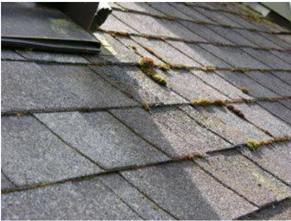
Photo 8-1 Moss growing on the roof. May require treatment.
