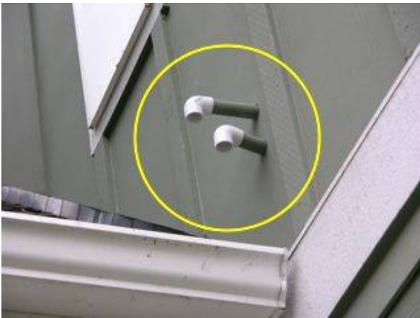
Photo 22-1 Temperature pressure relief valve piping can discharge to persons below.
